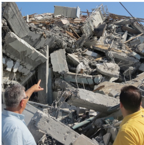
Destroyed Al-Wafa Hospital in Al-Shija'ia neighborhood, Gaza City. Surveying damages on the health sector.
